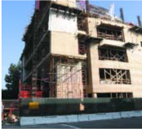
Trojan Founders Circle members visited the construction site of Ronald Tutor Hall, which is scheduled for completion in December 2004.
